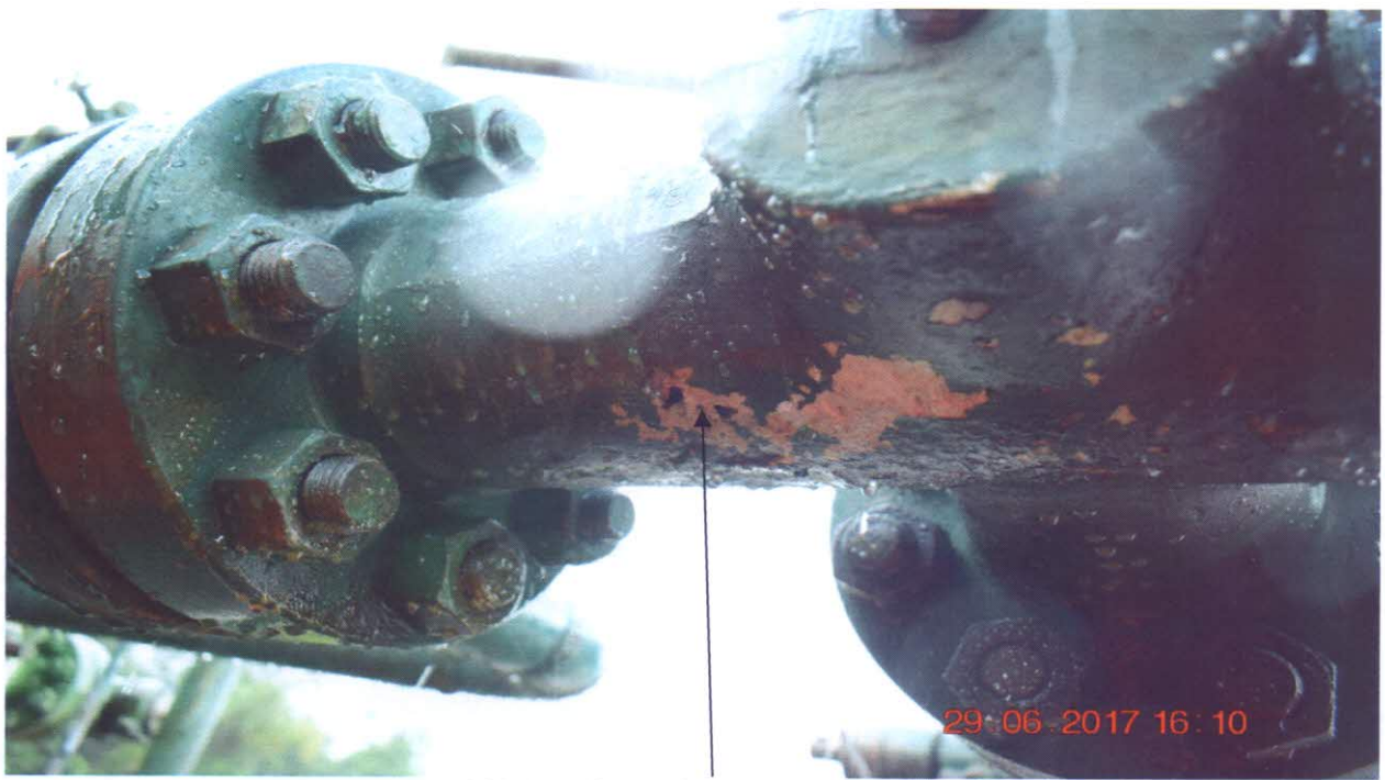
LEAK POINT (GOOSE NECK)
